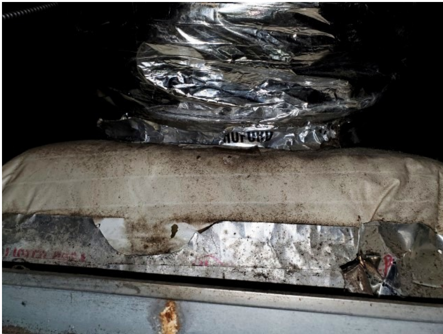
Photo 4: View of HVAC duct tape.
