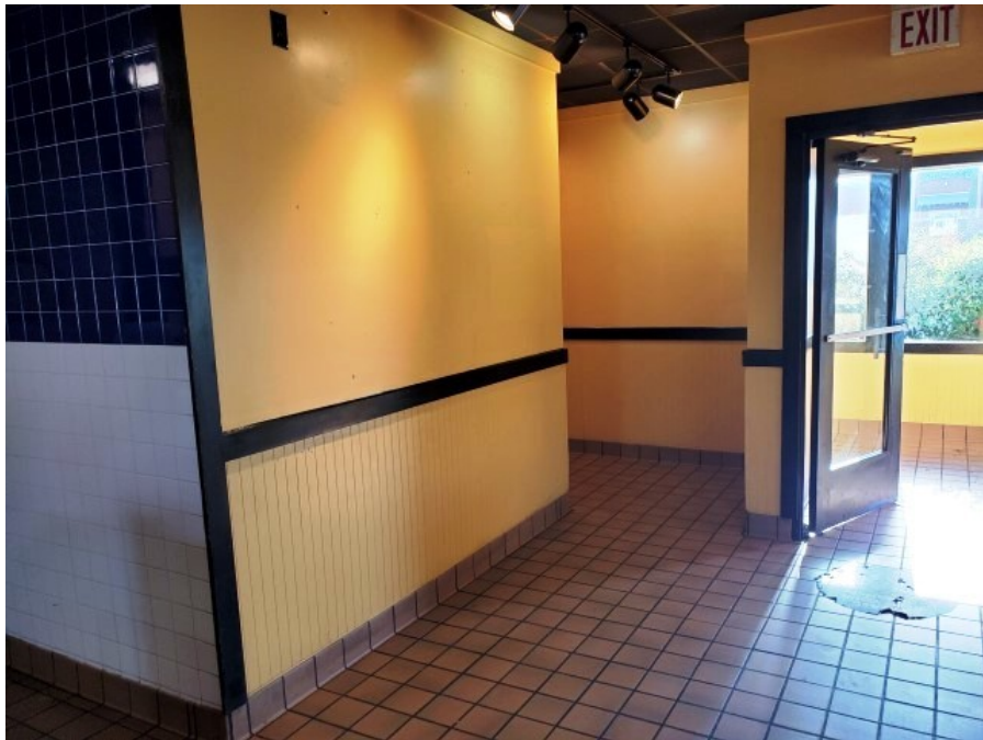
Photo 2: View of ceramic tile and wallboard systems.
