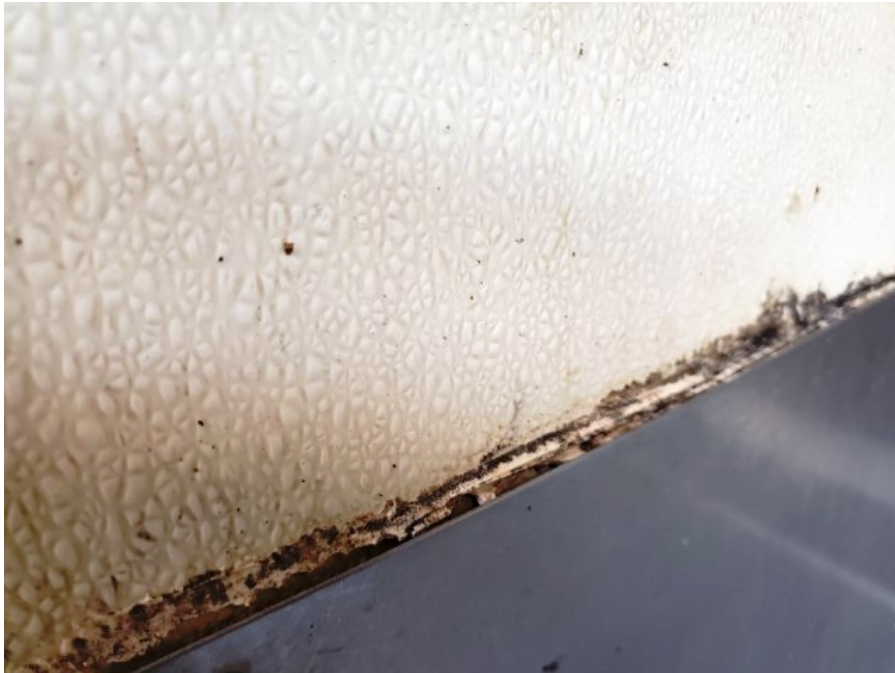
Photo 8: View of white kitchen caulk.
