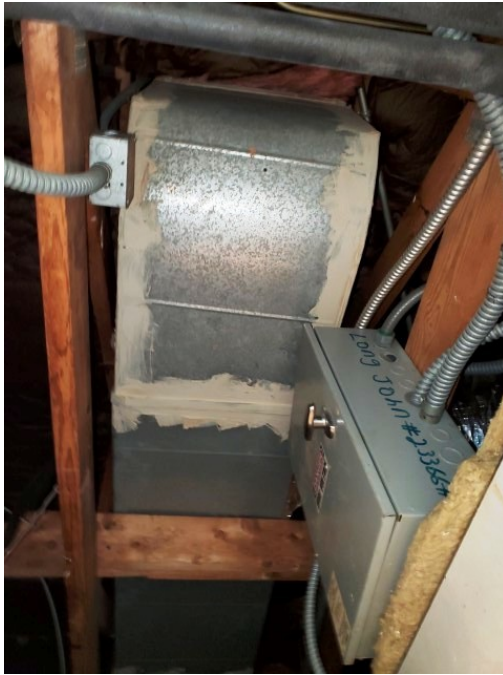
Photo 5: View of yellow duct mastic.
