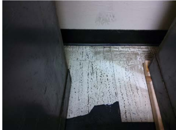
12-034, 035, 036 - 12"x12" White Floor Tile and Black Mastic
