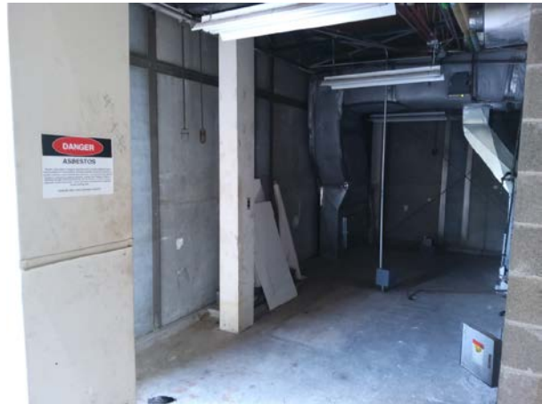
Mechanical Room 4, 2nd Floor
