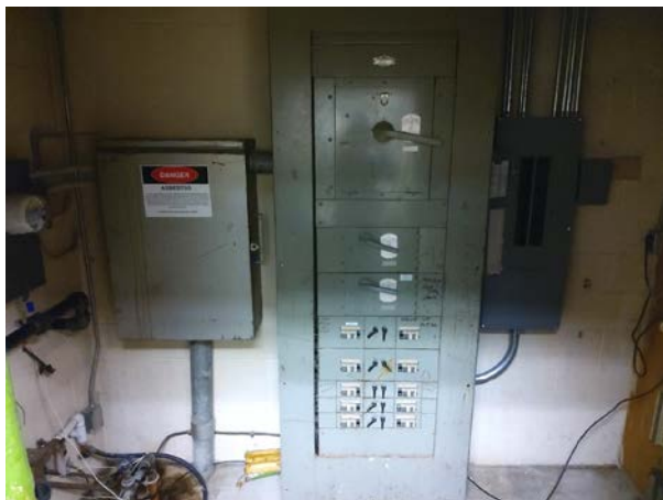
Mechanical Room 1, 1st floor
