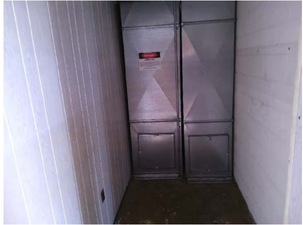
Mechanical Room 2, 2nd Floor
