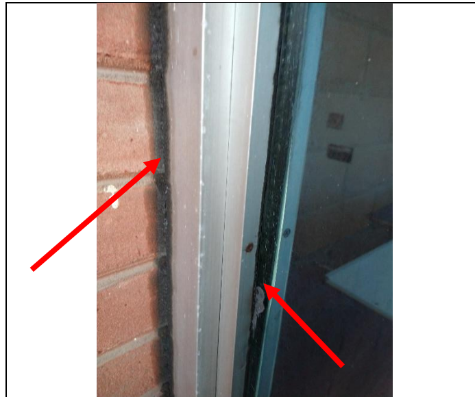
Photo #1 HA 17: Asbestos-Containing Gray Exterior Window Caulking/Glazing (2% Chrysotile)
