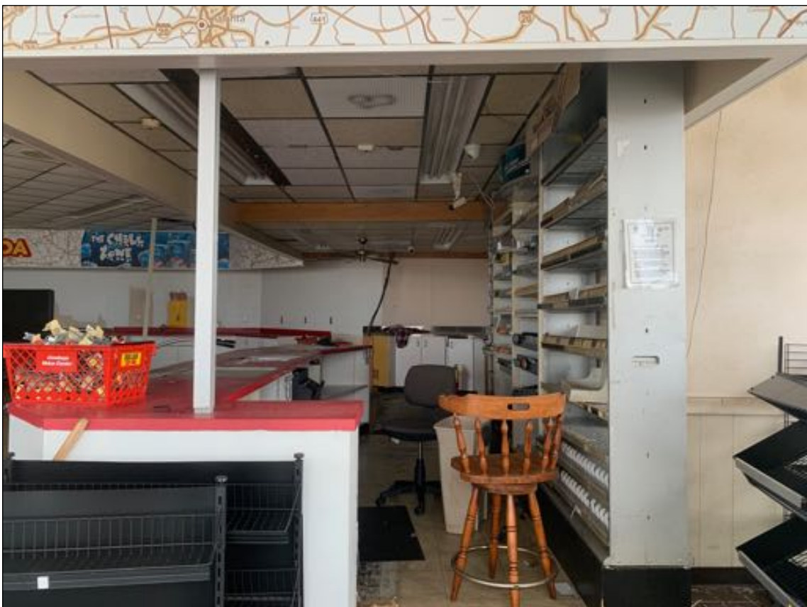
Looking inside the south-southwest end of the convenience store on the property
