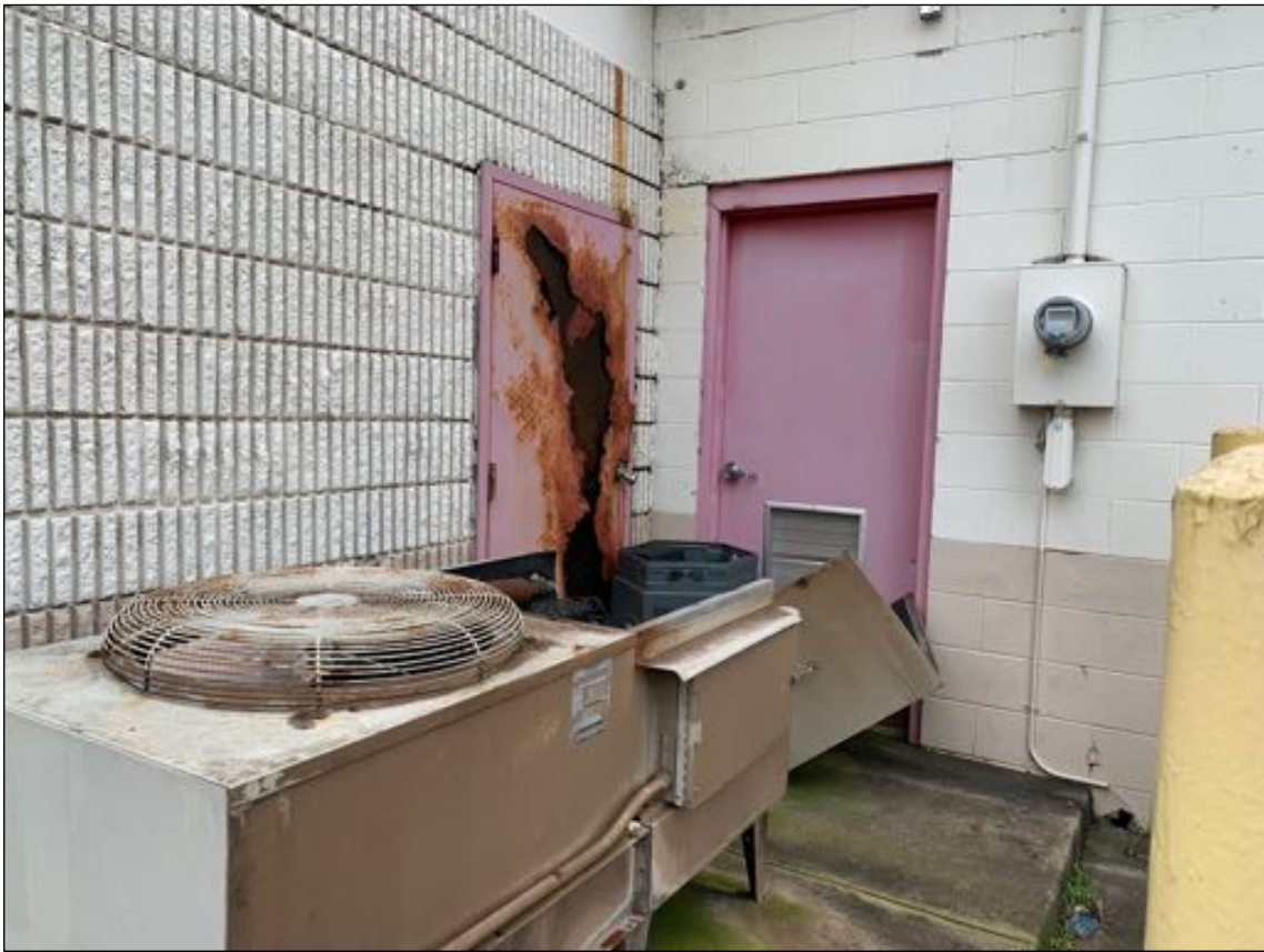
Looking at conditioning unit and back entrances at the northeast corner of the convenience store
