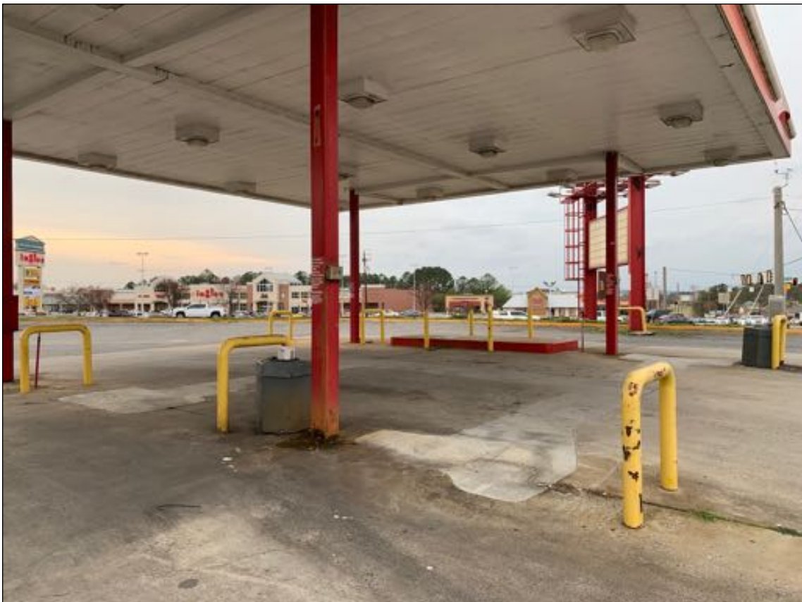
Looking at the former fuel pump island located on the Subject Property
