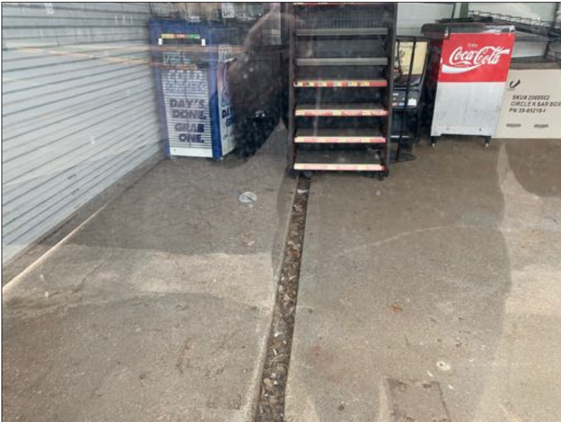
Looking inside the convenience store at the northeast portion of the building
