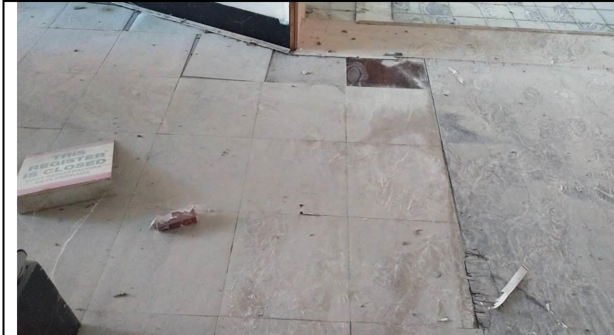
Photo 2: Non-ACM 12" X 12" Off White Floor Tile (HSM 02)
