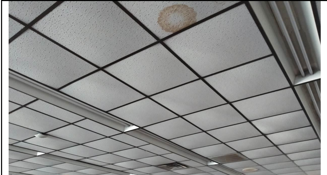
Photo 4: Non-ACM 2' X2 ' Fissured Ceiling Tile (HSM 04)
