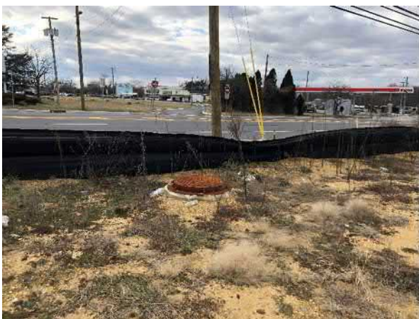
Photo 5 View of the sanitary sewer manhole on the southwestern portion of the site.
