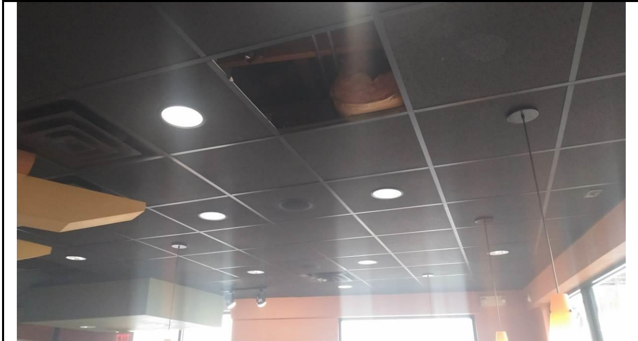
Photo 2: Non-ACM 2' X 2' Fissured Ceiling Tiles (HSM 02)
