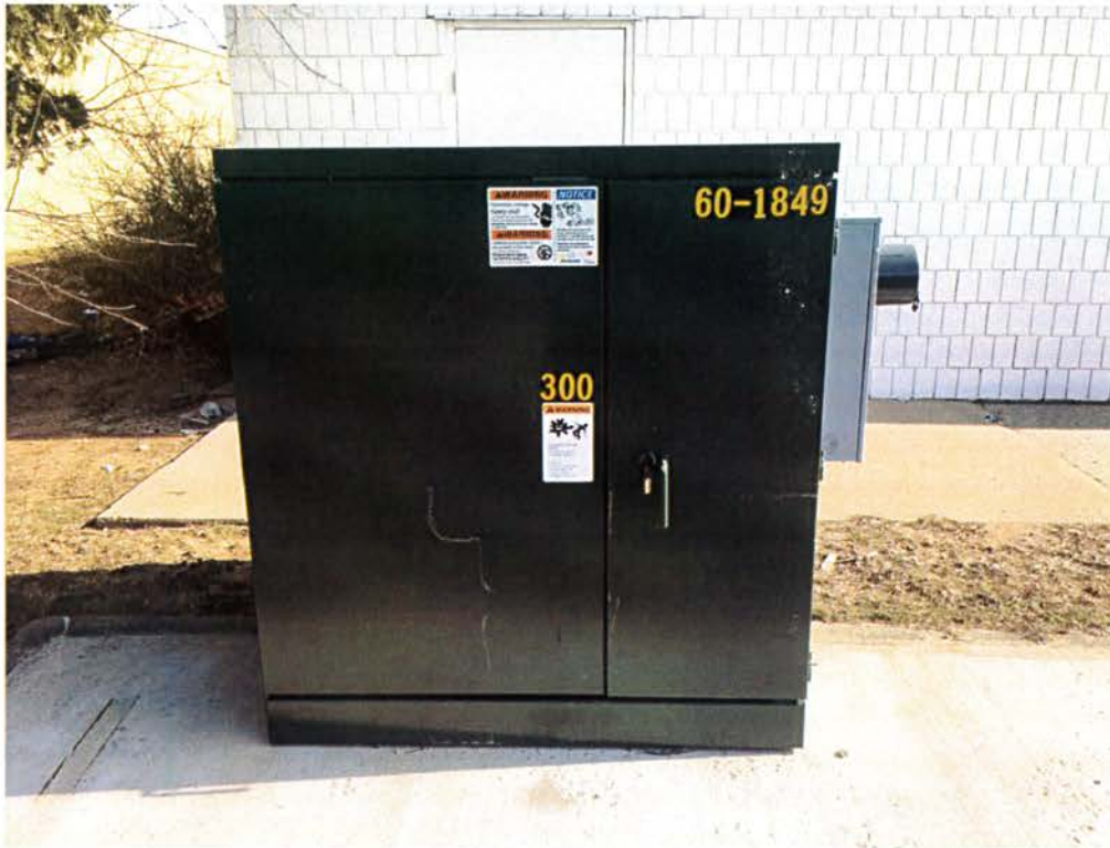
Typical Pad-Mounted Transformer
