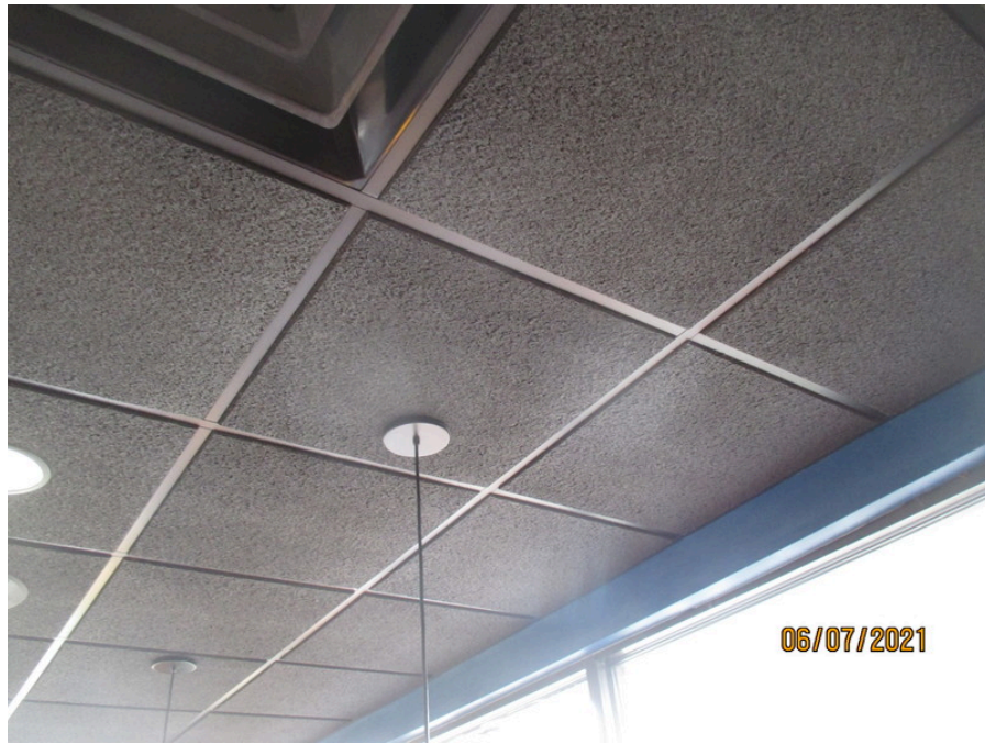
Photo 1: Non-asbestos containing ceiling tile, observed and sampled in the dining room (1A-1C)
