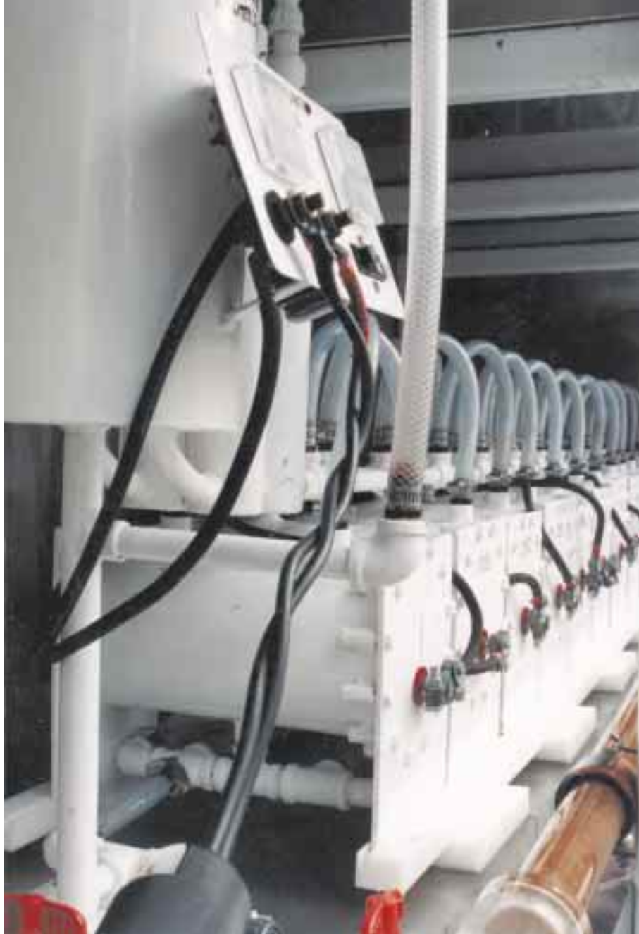
Above: Electrolyzers driven by photovoltaics.
